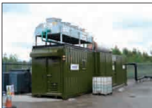
Figure 8.2 Landfill gas utilisation plant
