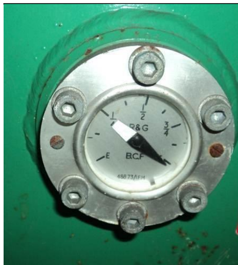
Photo 2: Halon Gauge Present on Cylinder
