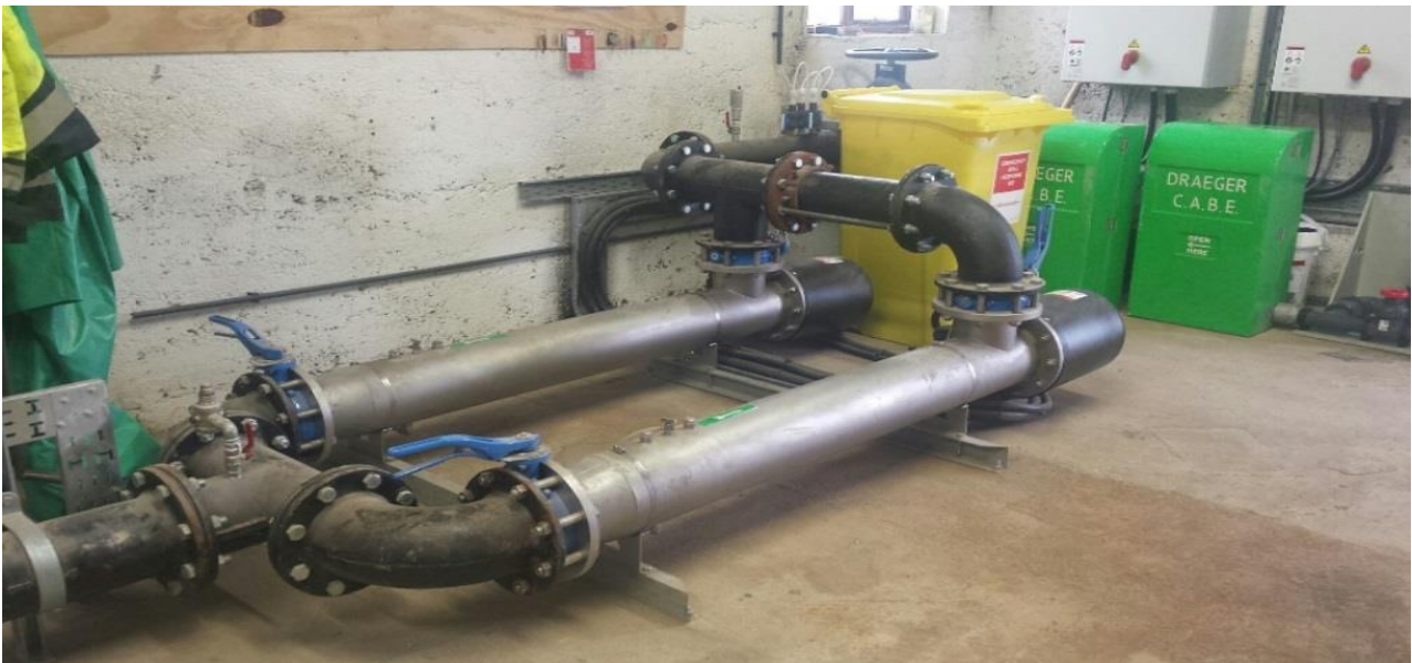
Figure 7: UV disinfection system
