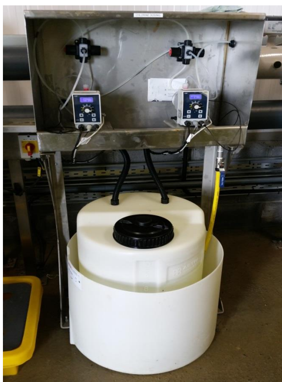
Figure 7: Sodium Hypochlorite disinfection system with bunded day tank and duty and standby dosing pumps
