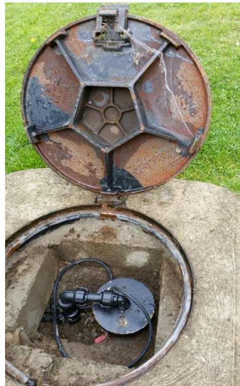
Figure 6: Borehole fully capped and sealed and in a locked chamber
