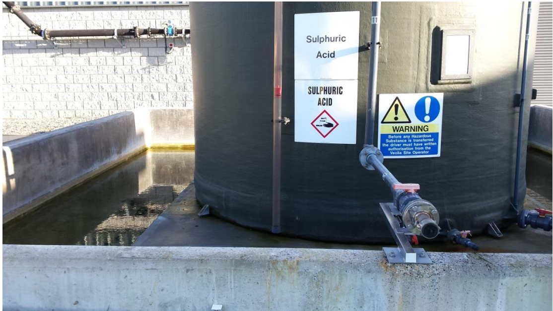
Photo 1. Sulphuric Acid Fill Point.
