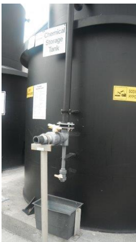
Photograph 1: Example of delivery pipe to bulk storage tank not within bunded area.
