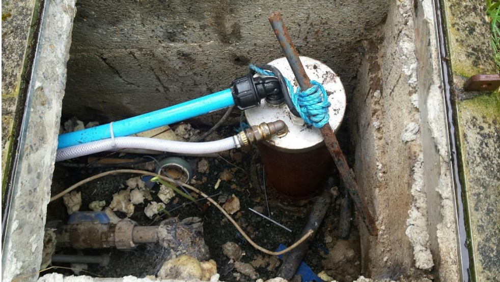
Photo 1: Ballingate Borehole (note the return water from the turbidity monitor being discharged back into the borehole via the white pipe).
