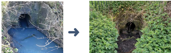
Outfall pipe to the river Griffeen before and after removal of domestic misconnections
