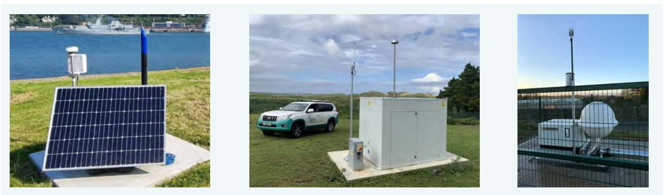
Figure 13. Equipment installed as part of the Network upgrade
