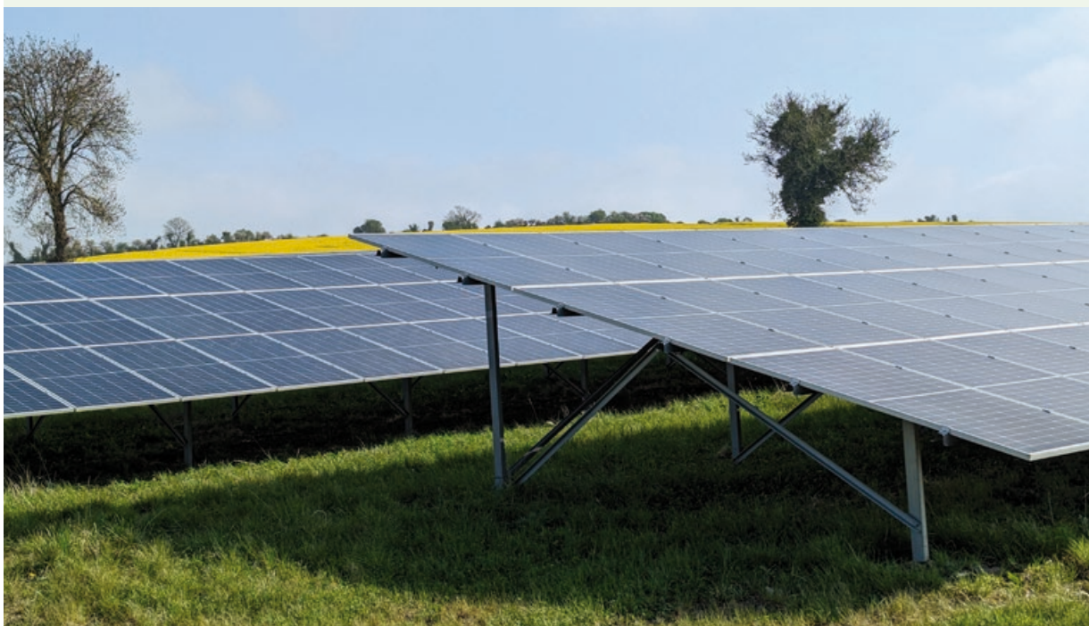
Figure 5.10 Solar array, Hilltown Solar Farm, Co. Meath
