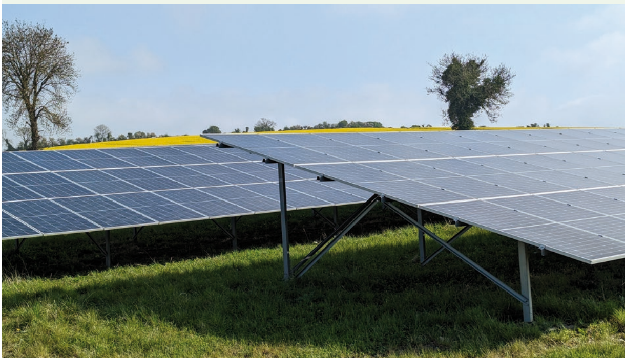
Figure 5.10 Solar array, Hilltown Solar Farm, Co. Meath
