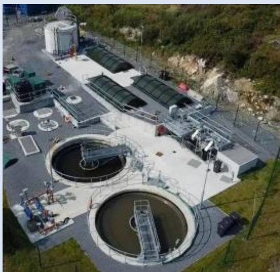
Figure 5: New wastewater treatment plant at An Spidéal
