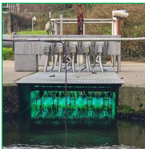
Figure 9: Ultraviolet disinfection system
